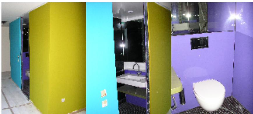
Figure 2: In-situ view of pod without glass sliding door (Courtesy: Sir Robert McAlpine)
