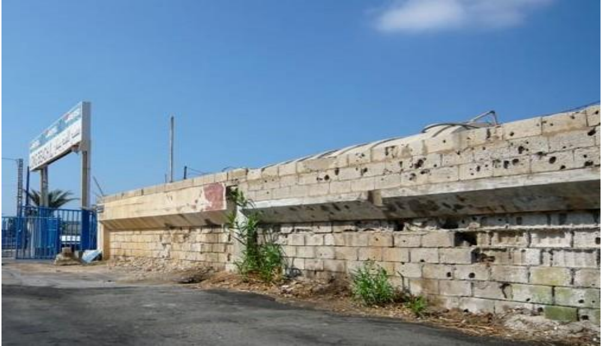
Fig. 12: Outer walls still bearing the scars of the Lebanese civil war 4
